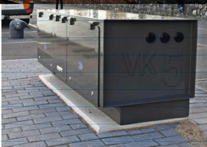
Ship to Grid charging point on Amsterdam dock
